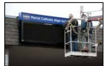
This Thursday, workers installed a new electronic reader board at the front of the school to replace the antiquated letter board. After years of waiting for the campus' zoning to be adjusted to allow for the sign, students were excited to see it installed at long last. Photo by Brennick Thompson
