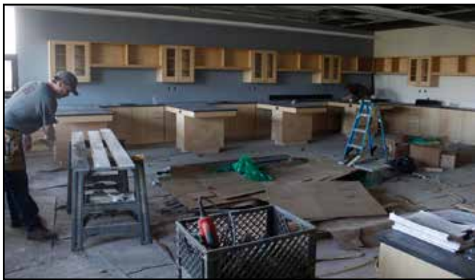
The finishing touches are added onto a science classroom. Photo by Toni Cooper
