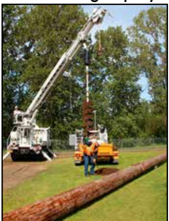
This week an osprey nesting station was installed on campus. It was installed in hopes of preventing the osprey from nesting at the track because the station currently installed at the south-west corner of the campus has been ineffective. Photo by Alex McQuaid '16
